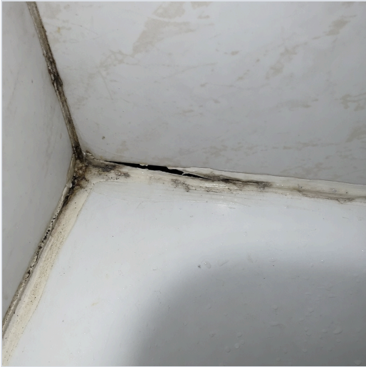
Photo 4. Tub surround, gap at tile joint.
