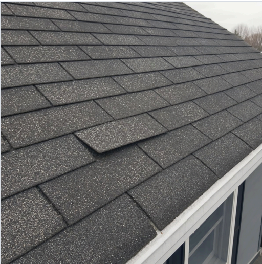
Photo 3. South slope, granule loss, lifted tab center-frame.
