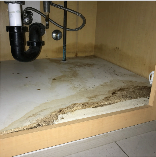
Photo 2. Kitchen sink cabinet, staining and swelling.
