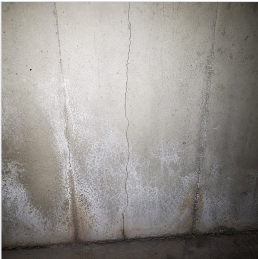
Photo 5. West foundation wall, hairline crack.
